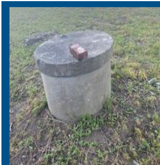
Old board well installed prior to 1990 Virginia Water Well Regulations
