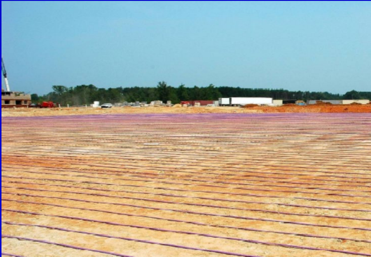
Purple Drip Wastewater Lines on Portion of Soccer Sports Field
