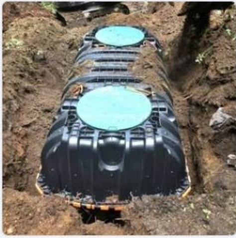
$1 Septic system Lexington, NC
