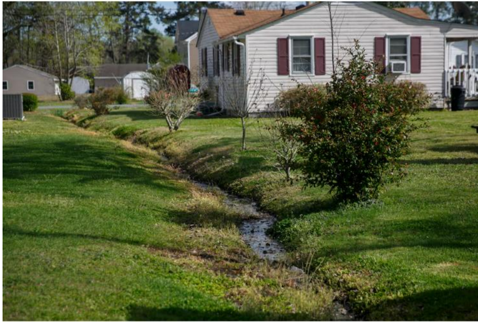
This trench was dug to help alleviate rainwater issues in the yard of Roosevelt Jones, whose septic system has increasingly failed at his Suffolk, Va., home. (Kristen Zeis for The Washington Post)
