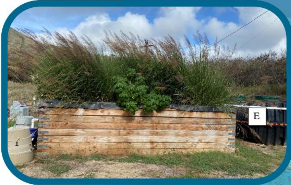
Bioreactor Garden + 1,000 Gallon Septic Tank (Infiltrator IM 1060)
